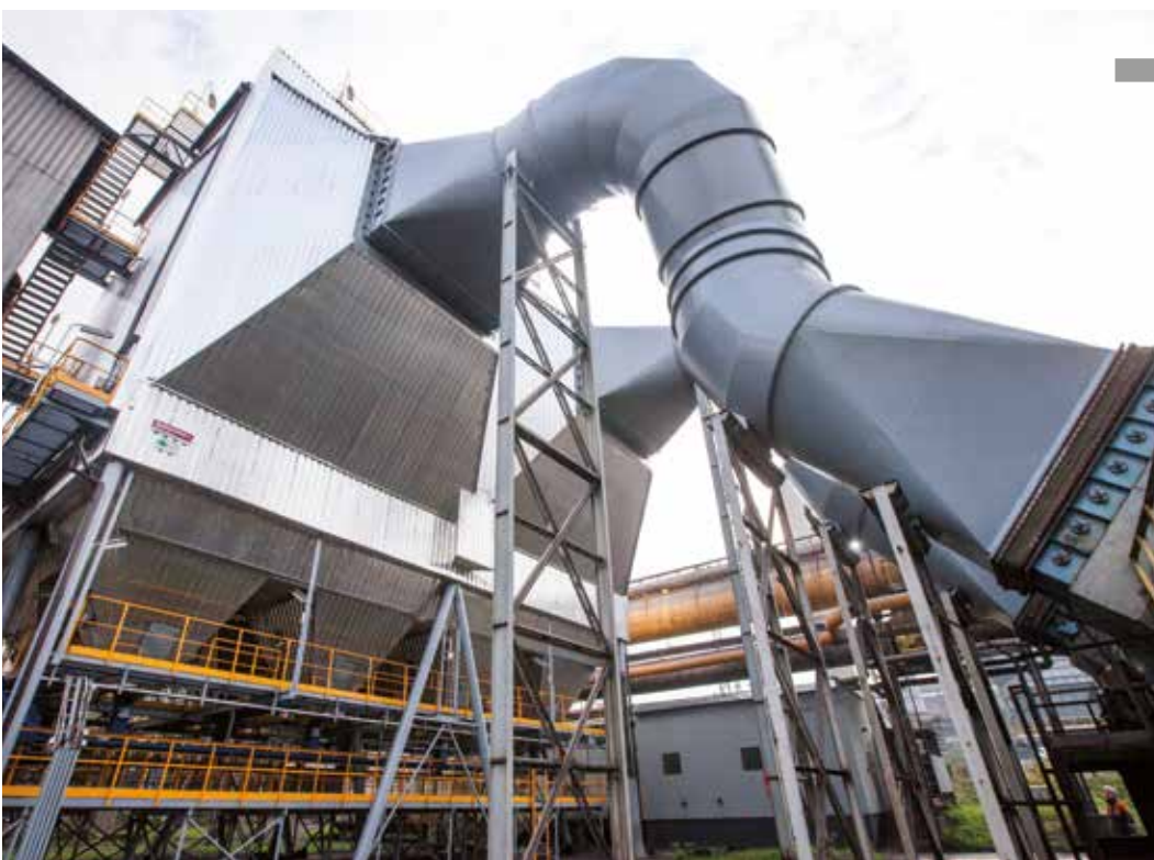
Elektrofiltr wielkiego pieca nr 5 w krakowskim oddziale ArcelorMittal Poland Electrofilter of Blast Furnace no 5 at Kraków unit of ArcelorMittal Poland
