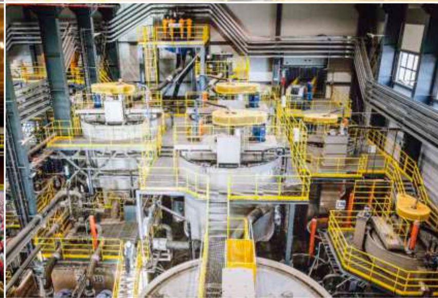
New flotation: flotation machines and tanks.
