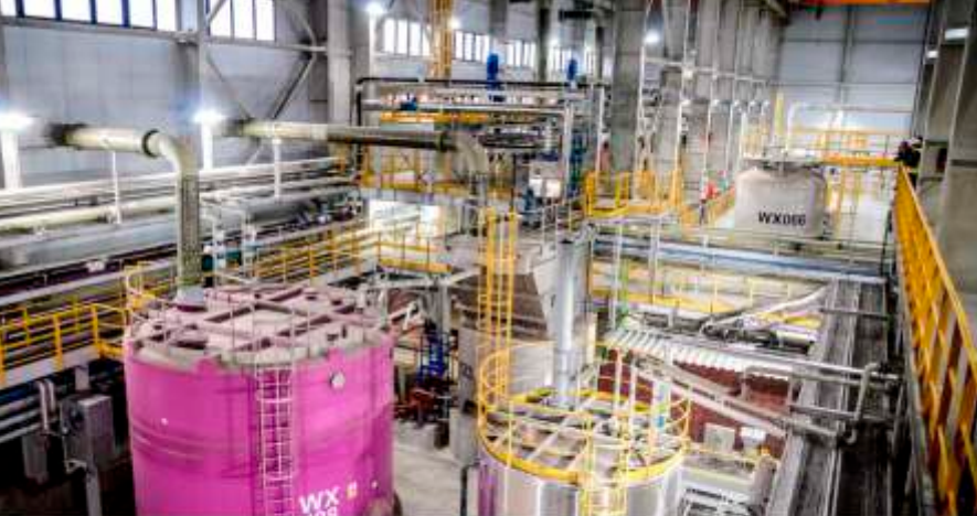
Waelz Oxide Plant: Front view of leaching ZnO oxide part. Tank WX 128 - \text{ZnSO}_4 solution.
